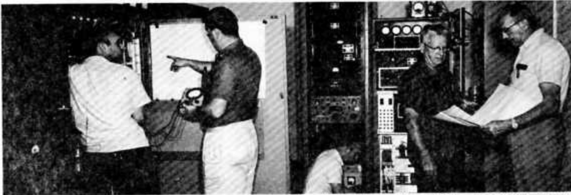
Shows installing the Ascension Island command control system that will be utilized on the next Saturn Launch, SA-6, are MTP personnel (from left) Harry Beatty, Sam Coble, Jackie Murphy, Stedman Chase and Russ Forsyth. SA-6 will orbit a "boiler plate" version of the Apollo spacecraft.
