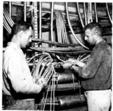
Range station wire technicians W. L. Andrus (left) and G. R. Wisman splice cable at the Cape Canaveral North Terminal Cable Building.
